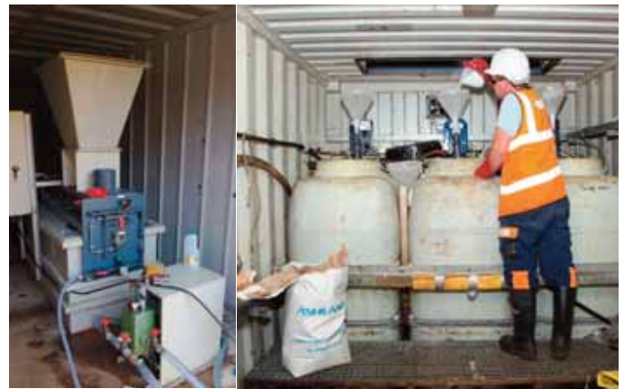
Above: Dosing station configured to requirements
