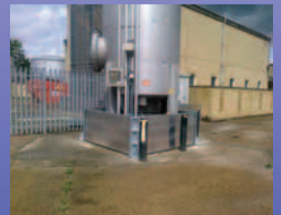
Demountable flood barrier around plant item
