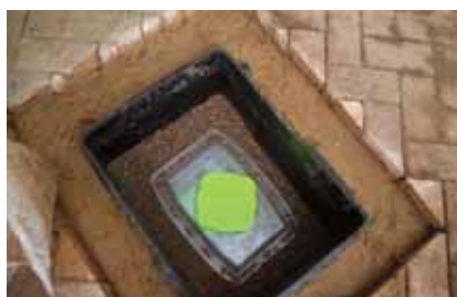
Flood Angel® 160mm/110mm Non-Return Valve installed underground
