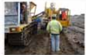
Cross Country Pipelines
