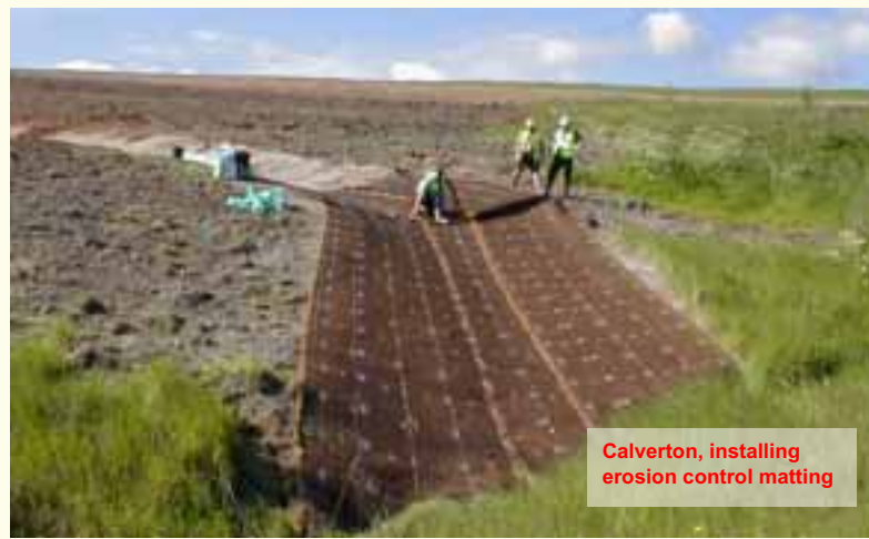
Typical surface water channel erosion damage with unreinforced soil at Calverton Notts
