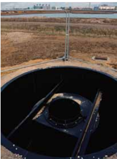
A Hydro Downstream Defender® providing the 2nd level of water treatment
